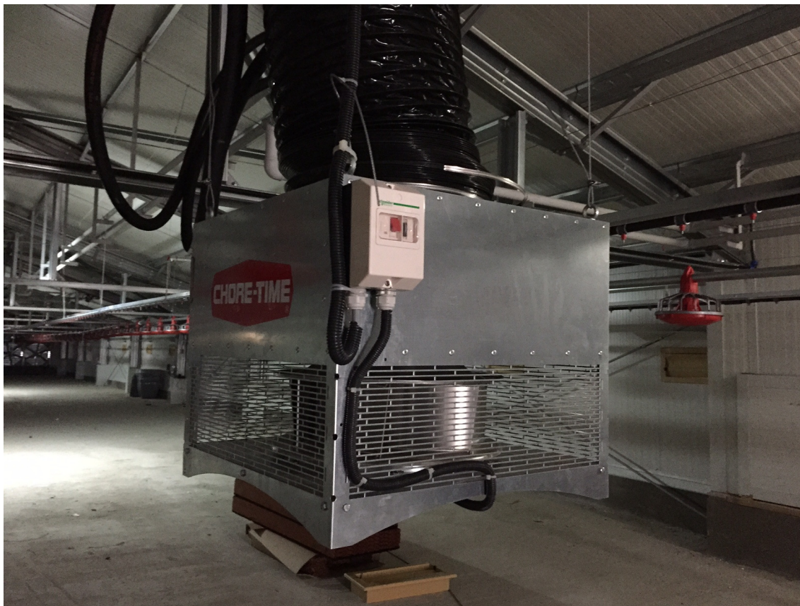
Termoconvector TUBO (hala noua)
