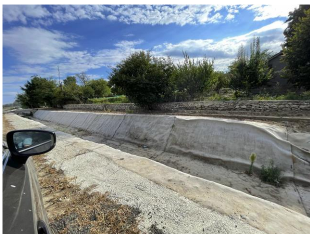
Colector SUD – degradat
