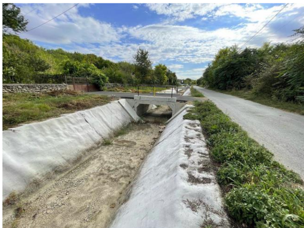
Colector vest – degradat
